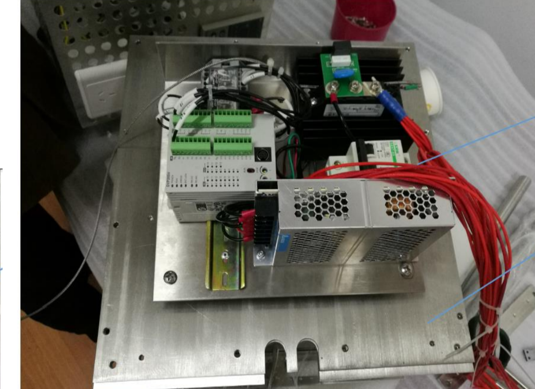
(e) Electrical Control System
